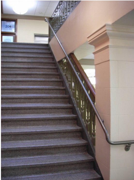
Stairs without handrails
